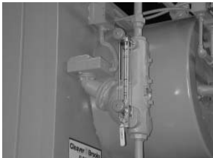
Figure 3-4: Low Water Cutoff and Gauge Glass with Blowdown Valve
