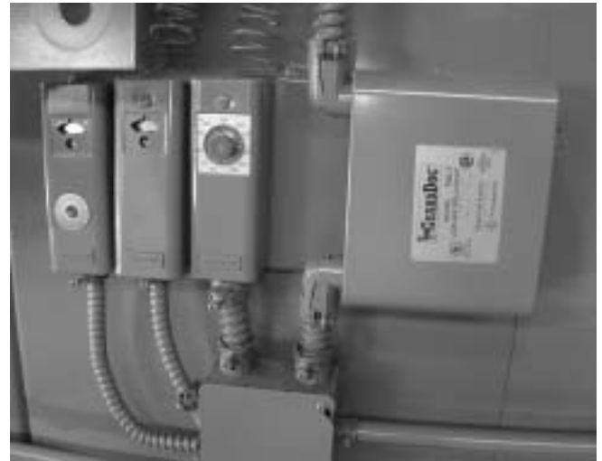
Figure 6-3: Hot Water Operating Controls
