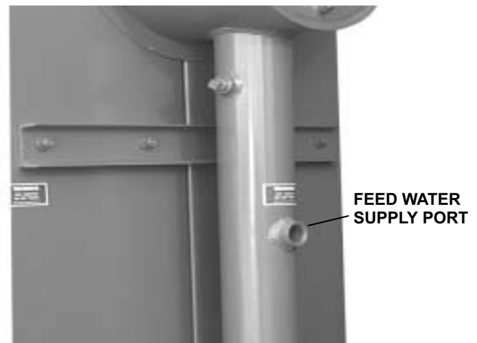
Figure 3-3: Feed Water Inlet Steam Boiler
