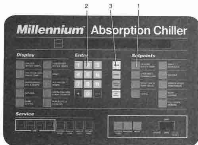
FIG. 4 - KEYPAD - PROGRAMMING "LEAVING CHILLED WATER TEMP" SETPOINT
