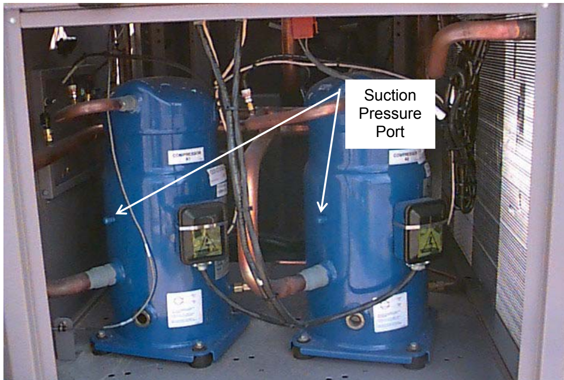
Figure 17 - Compressor Suction Service Port
