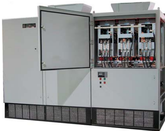
Fig. 12 – Front view of a 1750HP, 4160V drive with inverter section door open. Note roof mounted fans. There is room for a second set of fans.
