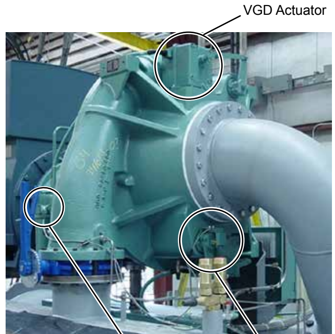
Transducer PRV Actuator VGD EQUIPPED COMPRESSOR
