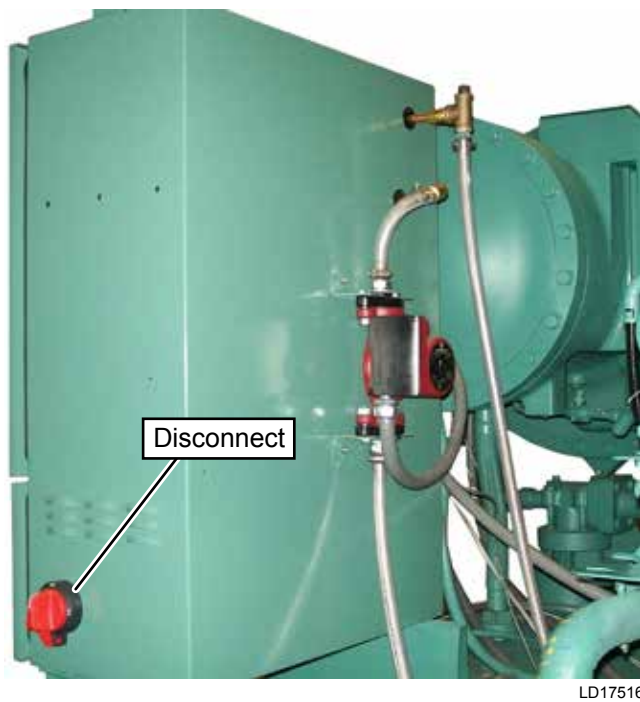
FIGURE 26 - POWER PANEL BATTERY DISCONNECT SWITCH
