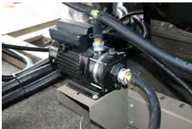
FIGURE 102 - VSD GLYCOL PUMP
