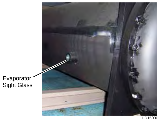
FIGURE 8 - EVAPORATOR SIGHT GLASS
