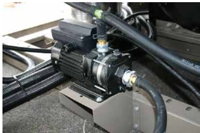
FIGURE 45 - VSD GLYCOL PUMP
